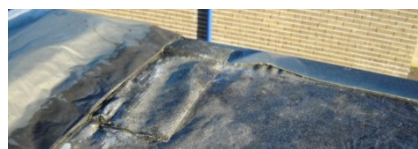
Defects require remedying
