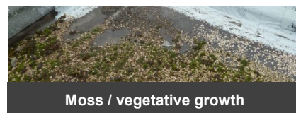
Loose / poorly adhered material
